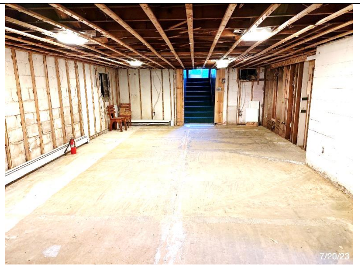
The basement family room with carpet, wall finish, and ceiling drywall removed by remediation firm; ready for a new look!
