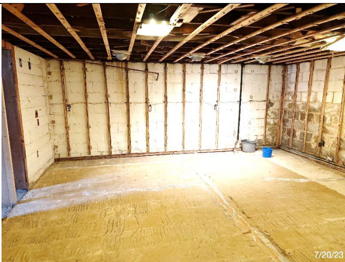
Basement family/recreation room – where the water finished its journey in the house.
