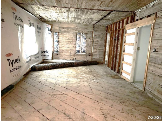
The Living Room after water remediation.
